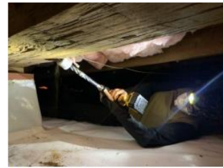
University of Louisville student Ginan Kurdi collects a core from a beam in the crawlspace of the Sandifer House.
